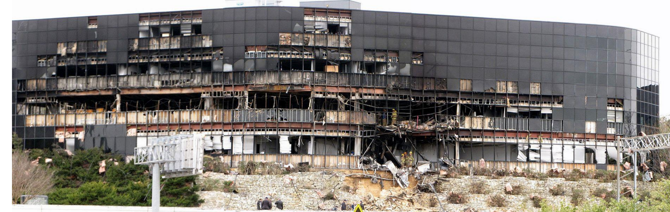
Austin, Texas, February 18, 2010. Single engine aircraft impacts the IRS Building killing 2 (pilot and one occupant of the building).
